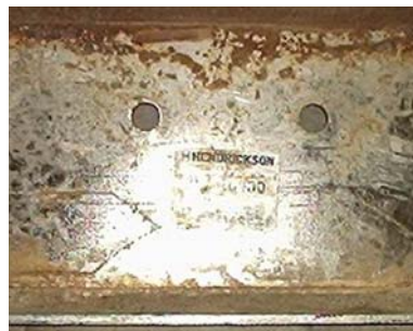
Corrosion on back side of the bumper
