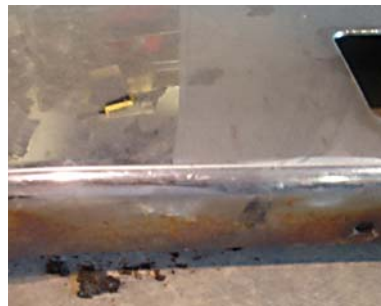
Corrosion on bottom flange of the bumper
