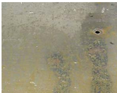
Orange / yellow corrosion distributed in relatively large areas
